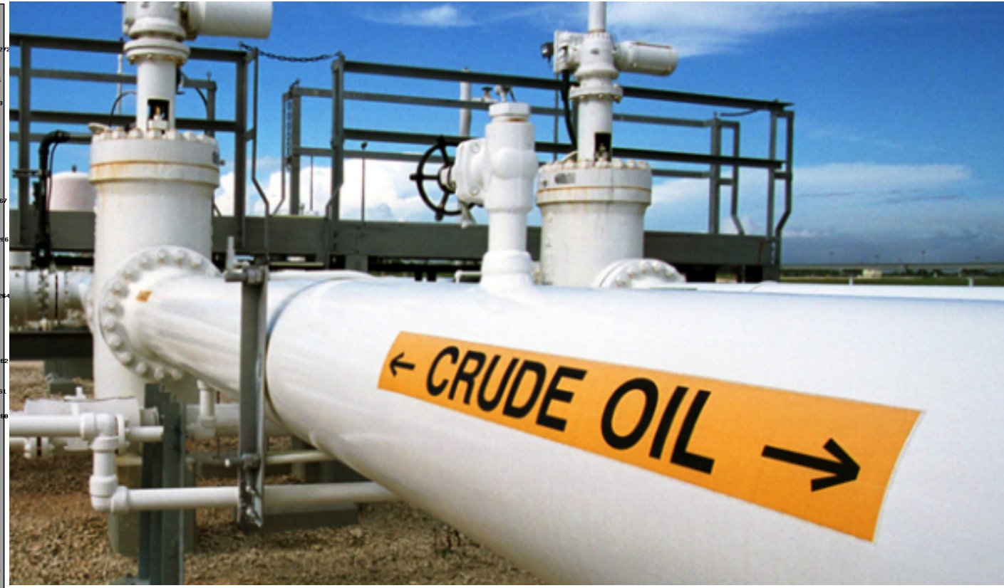
Crude oil pipeline, Texas photo credit Joe Raedle/News-makers via getty Images
